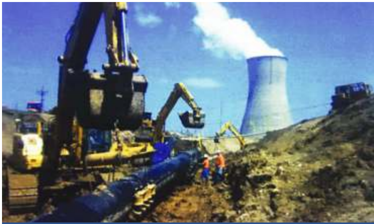
INDUSTRIAL PLANTS USING HDPE PIPE
